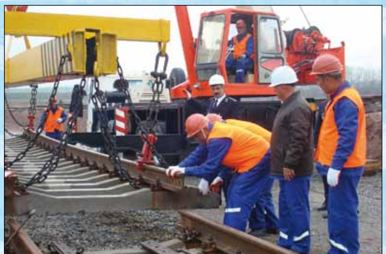
Laying down the first track section of Yavan – Vahdad railway line (Tajikistan)
