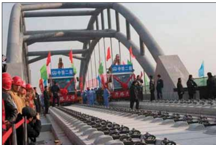
Final stage in the construction of high-speed railway line between Peking (Beijing) and Tianjin (KZD, China)
