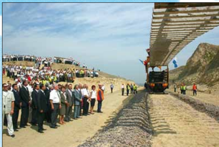
Ceremony of laying the last rails in a new track, constructed between Cahul and Giurgiulesti (Republic of Moldova)
